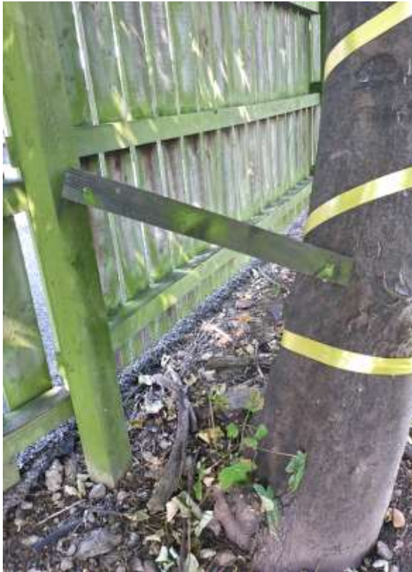
25. Remove fence support strut which is damaging tree.
