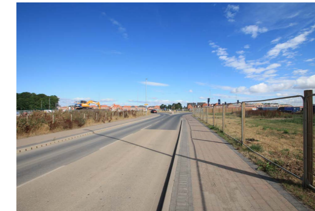
Works to footpaths, road connections, and bus stops have already been completed.
